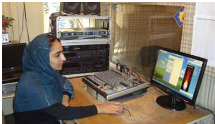
Control room at Radio Zohra, Kunduz
